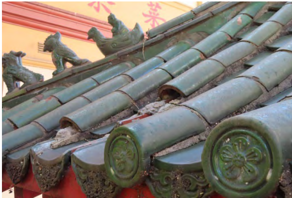
Figure 4.41 Some broken tiles on the eastern bay.
