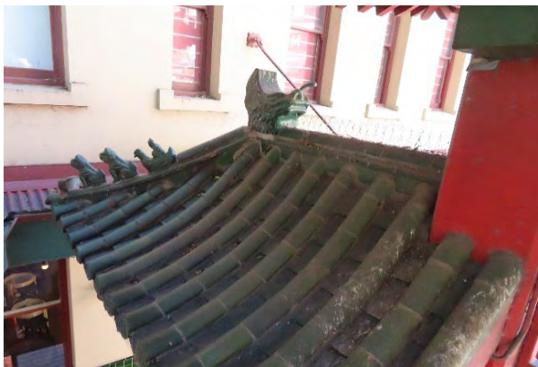
Figure 4.37 Roof tiles in fair condition. Note parts of the decorative ceramic figures are broken.
