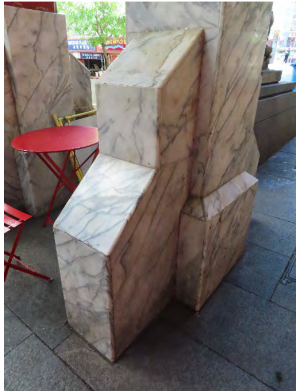
Figure 4.27 Chipped marble plinth.
