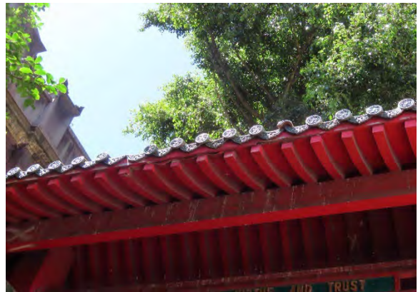
Figure 4.19 Missing/broken ceramic tile on the upper roof above the main beam.
