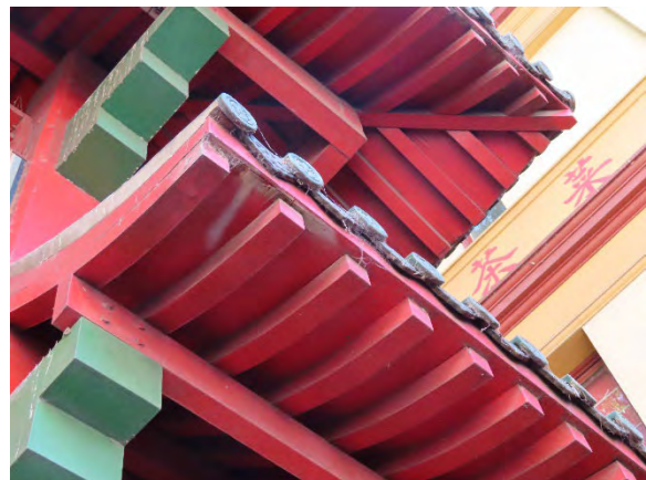
Figure 4.44 View of the underside of the upper and lower roofs showing delaminating plywood soffit.
