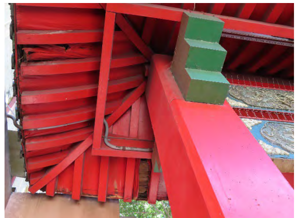
Figure 4.48 Deteriorated timber rafter and damaged plywood soffit.
